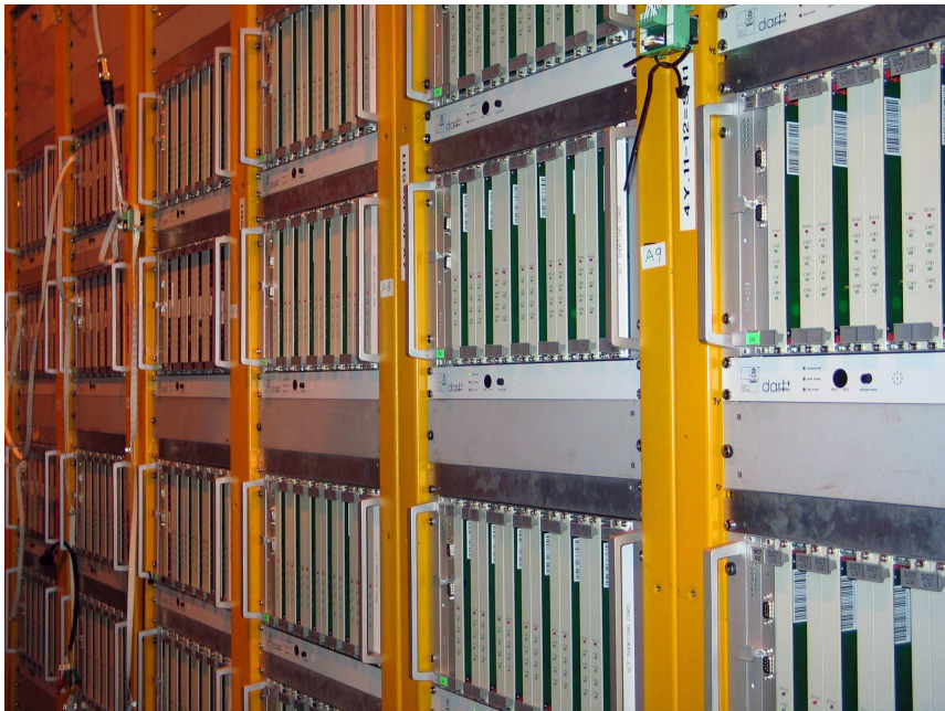
Power supplies in SR1.
